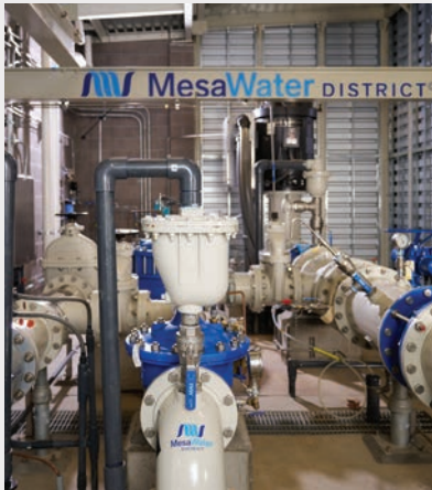
One of Mesa Water's newest groundwater wells that pumps 4,000 gallons of local, clean, safe water per minute.
