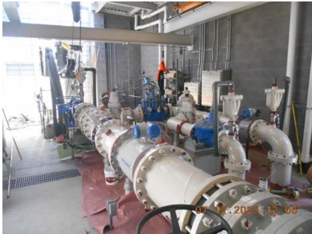
Figure 1. Well No. 12 Wellhead Piping
