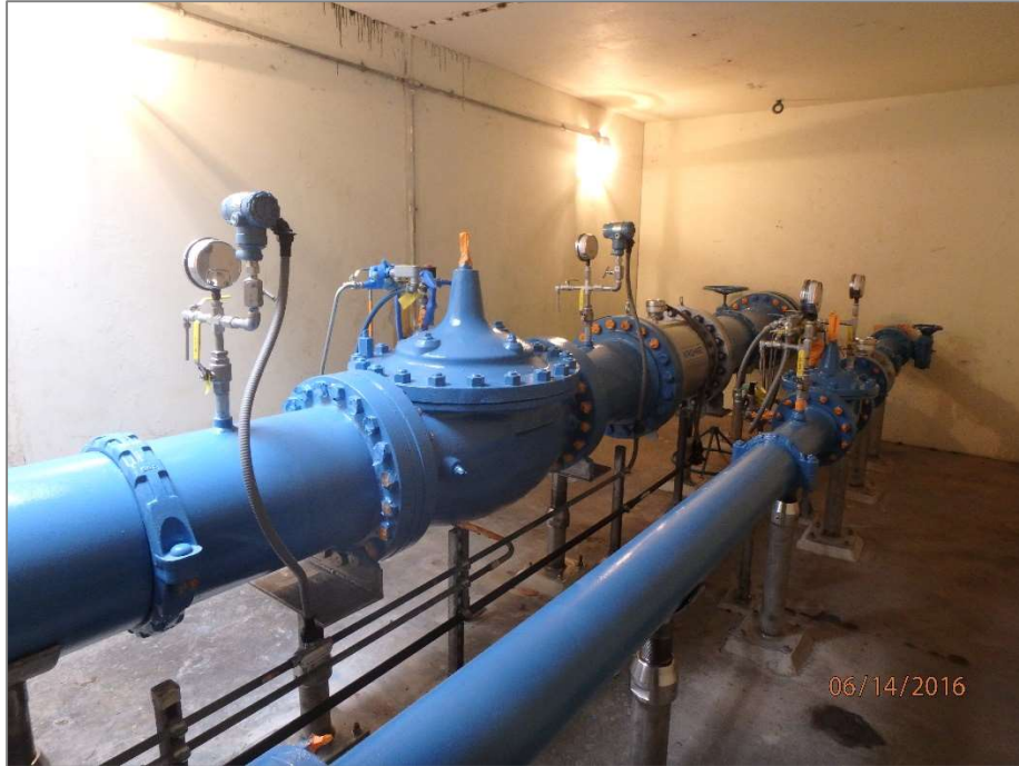
Figure 4-6. Photograph of OC-44, Sub-Turnout 4
