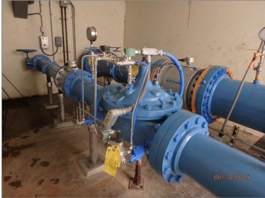
Figure 4-4. Photograph of OC-44, Sub-Turnout 2
