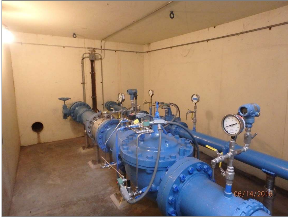
Figure 4-8. Photograph of OC-44, Sub-Turnout 5
